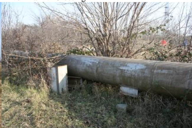
Aboveground Section with the Damaged Supports
