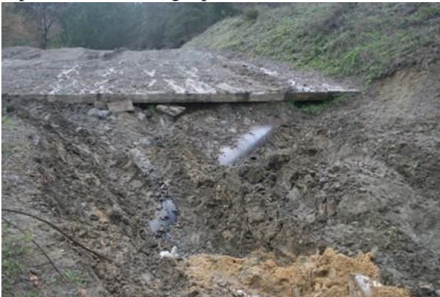
Damaged Road Crossing
