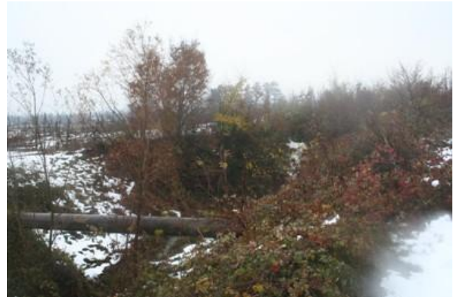
Exposed Pipeline across the Gully Crossing
