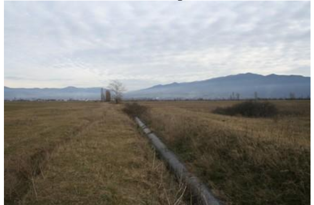
Exposed Pipeline in the Poorly Backfilled Trench
