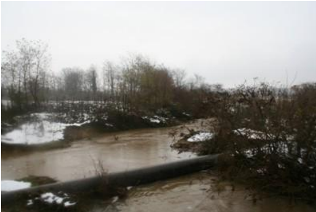
Exposed Pipeline in the River Rushava
