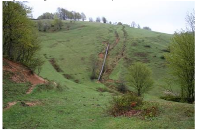
Pipeline Section in a Heavily Eroded Area
