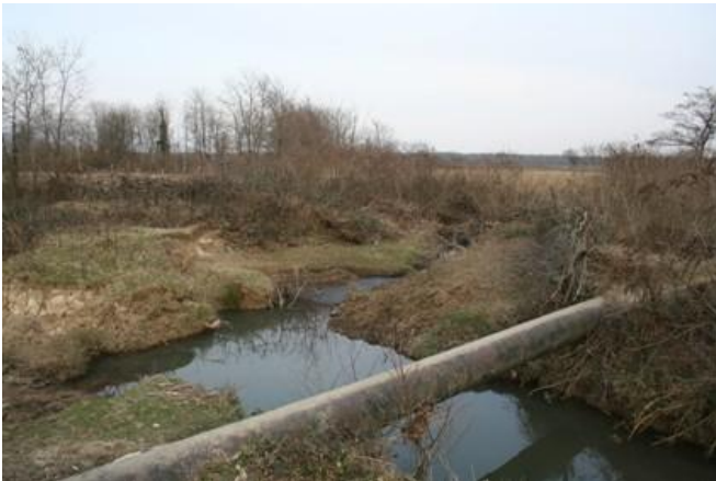
Exposed Pipeline across the Eastern Tortla
