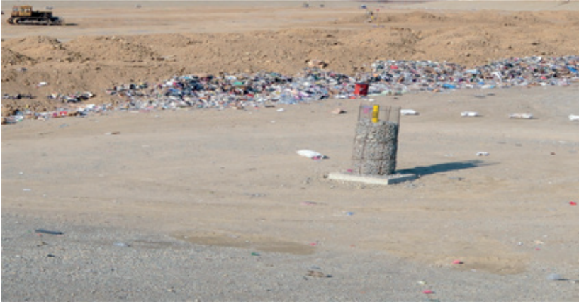
Photo 6.2.2.1. Part of methane collection system mounted at the Tbilisi new landfill
