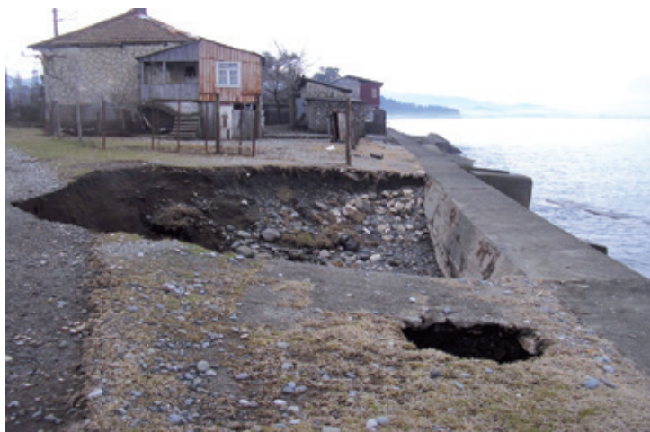
Photo 6.1.3.1. The funnel-form cavity washed out by the wave behind the wall
